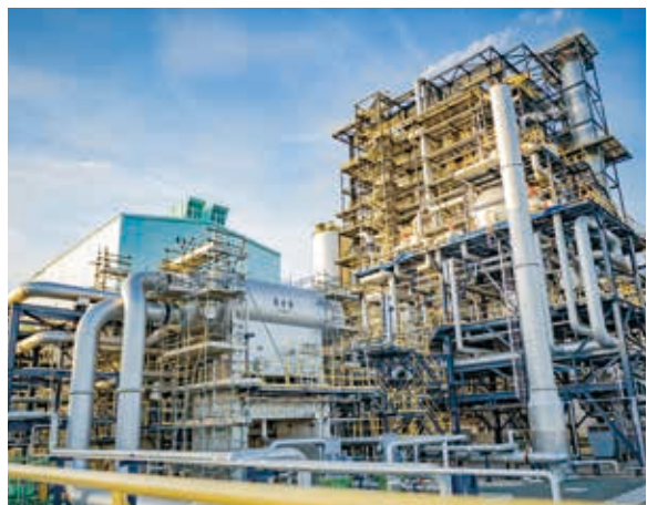
Biomass Power Plant (Japan)
