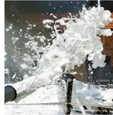
Foam Extinguisher System
