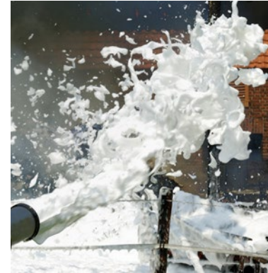
Foam Extinguisher System
