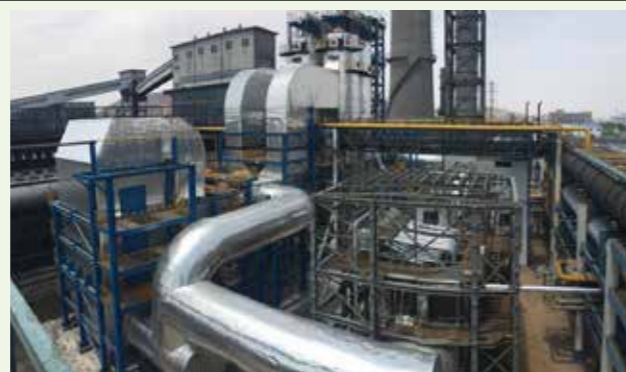
Dry-type SOx and NOx removal system for mid- and low-temperature flue gases installed at coke manufacturing plant (Inner Mongolia Autonomous Region, China)
