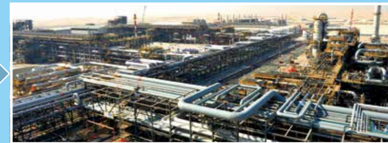
Plant facilities constructed by JGC
