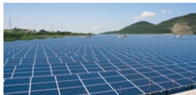
Mega-solar power plant for Futtsu Solar, Inc. (Chiba, Japan)
