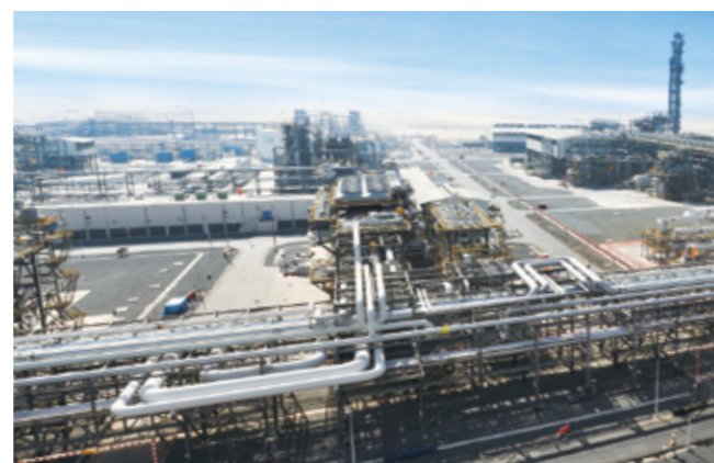
A large gas processing plant under construction for Abu Dhabi Gas Industries (Emirate of Abu Dhabi, United Arab Emirates)
