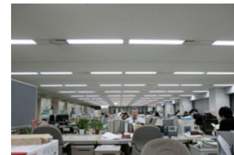
LED lighting in the office floors of the Company's Yokohama World Operations Center
