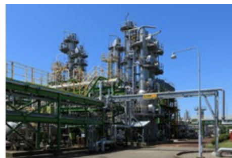
Koshijihara Gas Plant of INPEX Corporation
