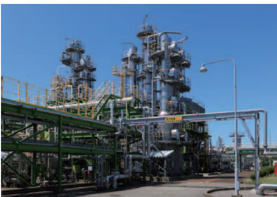
Koshijihara Gas Plant of INPEX Corporation
