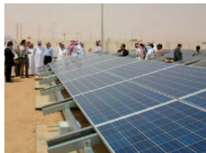
Visit to the solar photovoltaic power generation demonstration facility in Saudi Arabia
