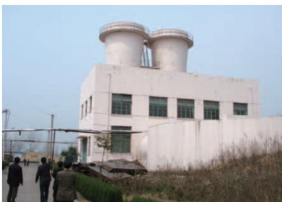
Coal mine VAM duct
