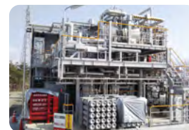
Ammonia synthesis pilot project facility (Fukushima)
