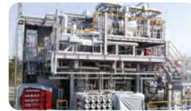
Ammonia synthesis pilot project facility (Fukushima)
