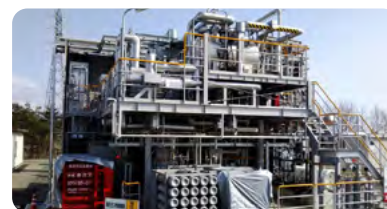
Ammonia synthesis pilot project facility (Fukushima)
