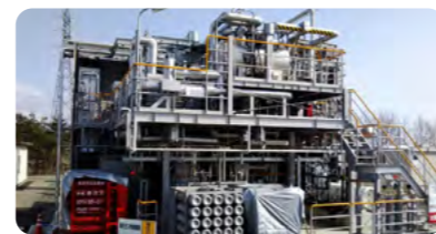
Ammonia synthesis pilot project facility (Fukushima)
