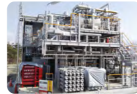
Ammonia synthesis pilot project facility (Fukushima)
