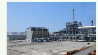
Site for the Construction of Domestic SAF Manufacturing Equipment (Sakai Refinery, Cosmo Oil Co., Ltd.)
