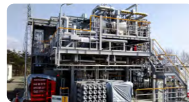
Ammonia synthesis pilot project facility (Fukushima)
